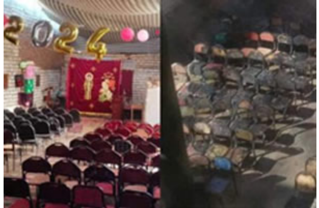
The temporary church building before and after the arson attack. Photo: Christian Solidarity Worldwide
